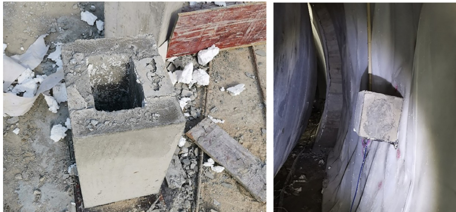
Fig. 10. Embedded structural defects in the tunnel lining at the physical testing site.
