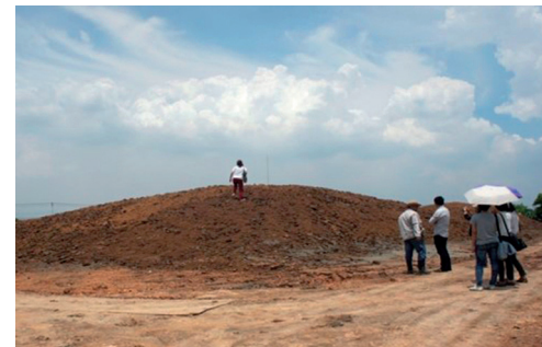
4th Month: Sculpted berm topped with a 1-meter deep mixed soil 第4个月：塑造出的坡地之上覆盖有一米高的混合土
