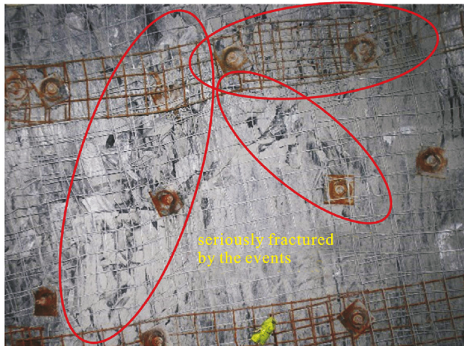
Fig. 12. The wall of a mine stope reinforced with Type 2 support method GDS system immediately after the second seismic event of two subsequent events 2.9 and 2.2 Mn, respectively. (Courtesy of D. Counter).
