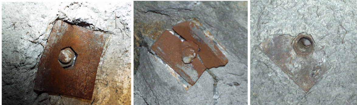
Fig. 22. Premature failure of plates and thread of the rock bolts.
