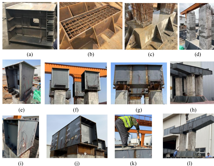
Fig. 6 The fabrication process of specimens: (a) fabrication of steel cap beam segments by welding steel plates; (b) the rebar framework of the concrete foundation; (c) the rebar framework of the concrete column and the cast concrete of the foundation; (d) concrete casting of the columns. Specimen S1: (e) installation of the cap beam–column joint segment with the bolts between the webs tightened; (f) installation of two joint segments; (g) welding of the segments between columns, casting of UHPC, and tightening of bolts on the outer sides of webs; (h) The complete specimen S1. Specimen S2: (i) installation of the cap beam–column joint segment; (j) welding of the segments between columns; (k) casting of the concrete at the joints; (l) the complete specimen S2.
