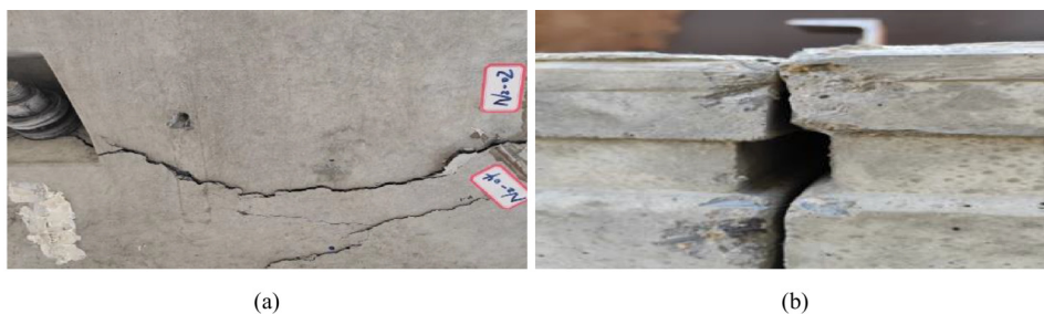
Fig. 8 Overall damage of the joint: (a) hand hole for curved inner surface; (b) outer curved surface contact.
