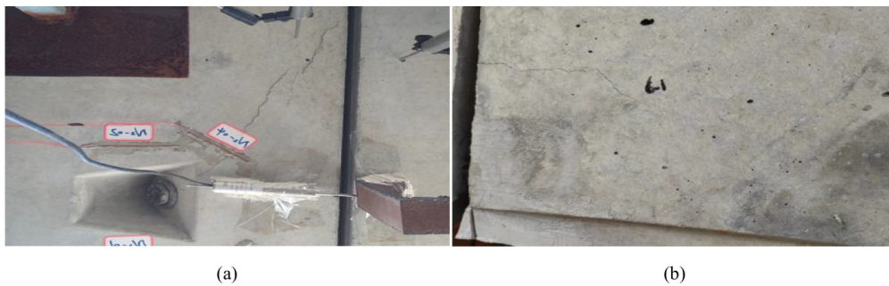
Fig. 7 Inner arc cracking stage damage: (a) inner curved surface hand hole cracking; (b) side concrete cracking.
