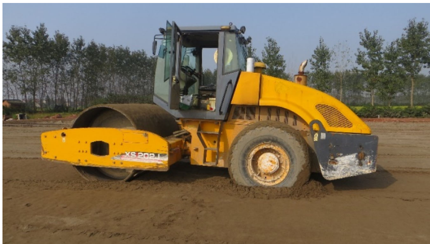
Fig. 5 Vibratory roller of 22 ton was stuck in wet sand when compacting
