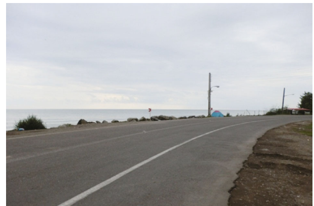
Fig. 3 Coastal road exposed to waves
