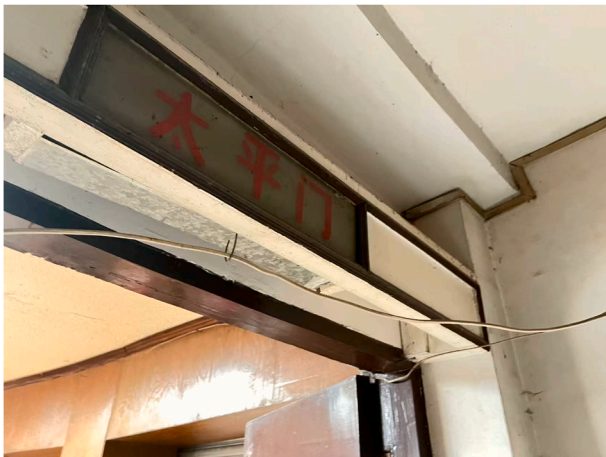
Fig. 19 The evacuation sign.
