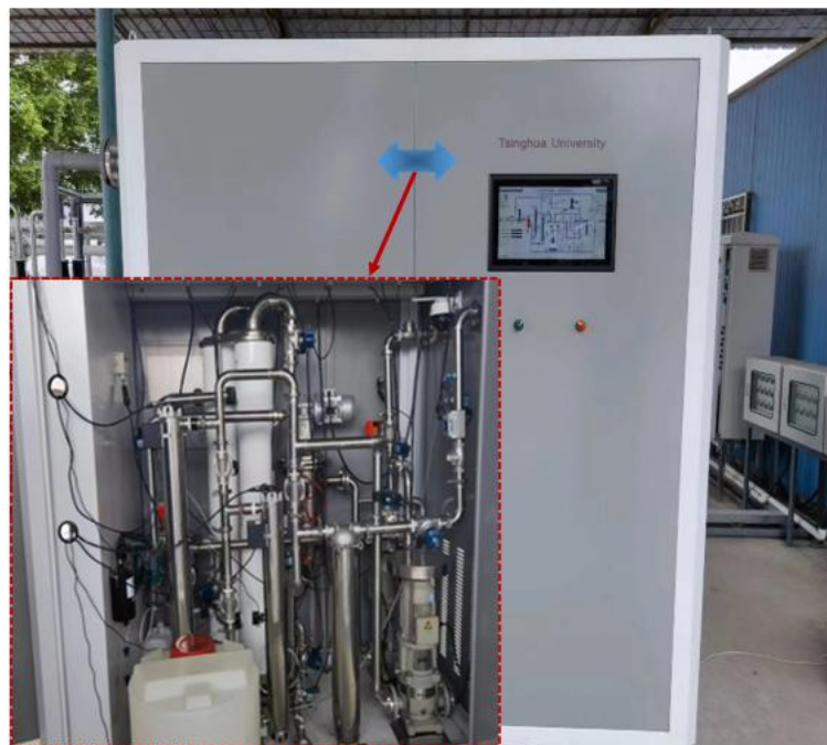
Fig. S1 The UV/H 2 O 2 advanced oxidation integrated pilot water purification system.
