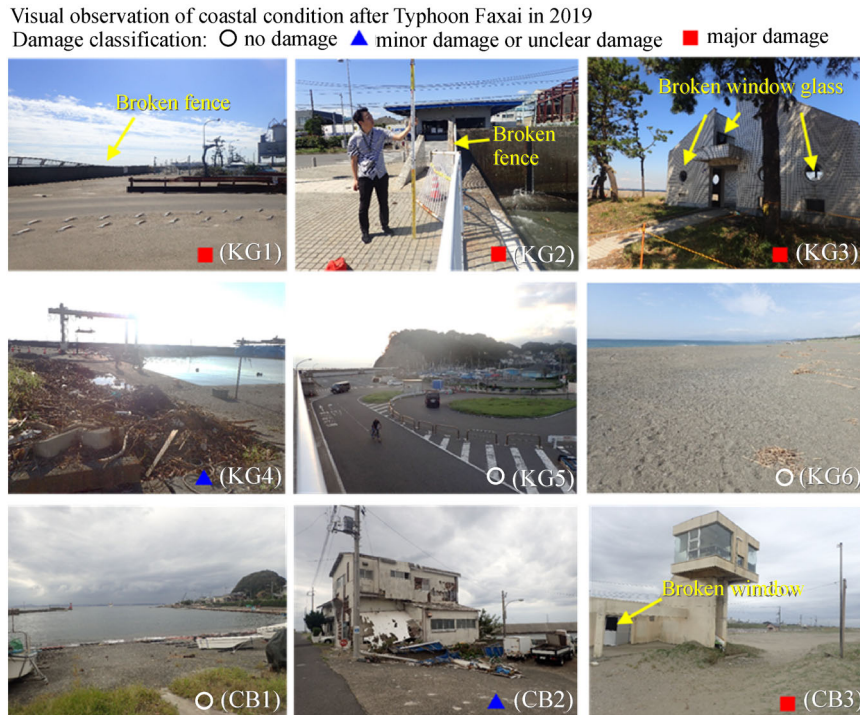
Fig. 3 Scenes after Typhoon Faxai in Kanagawa and Chiba prefecture (all photos taken by the authors). Minor damage: objects are scattered or adhered, but there is no noticeable damage to the building or structure caused by waves. Major damage: Partial or total damage to the building or structure caused by waves.
