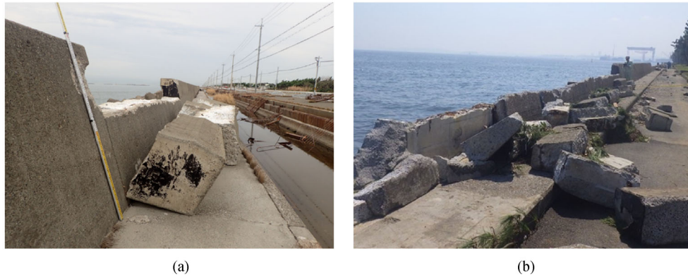
Fig. 1 (a) Failure of the coastal dike in Osaka, caused by high waves due to 2018 Typhoon Jebi (photo taken by the author); (b) Damage in Yokohama, due to 2019 Typhoon Faxai (photo courtesy of Port & Harbor Bureau, City of Yokohama).
