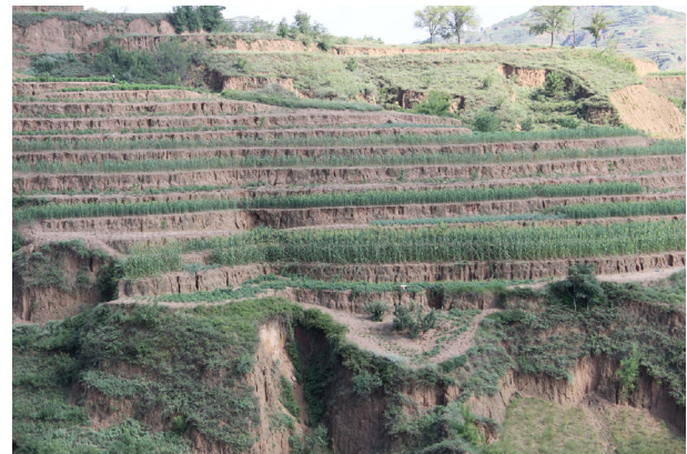
Fig. 15 Part of the terraces damaged in the Suide 7.26 heavy rainfall event in the Jiuyuanguo watershed (Photo taken by Qinke Yang on July 29, 2017).
