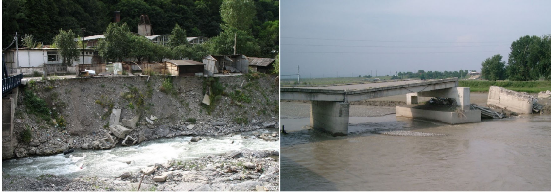
Fig. 4 Left: Buildings on the Prahova River at Comarnic, damaged by riverbank erosion as a result of the flash-flood of July 2005 (photo: Gabriela Ioana-Toroimac). Right: Bridge destroyed by the flash-flood which occurred on the Prahova River in July 2005, at Nedelea (photo: Liliana Zaharia).
