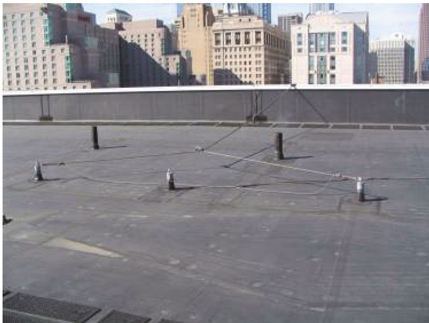
Figure 2. The safety rope anchors on the roof.
