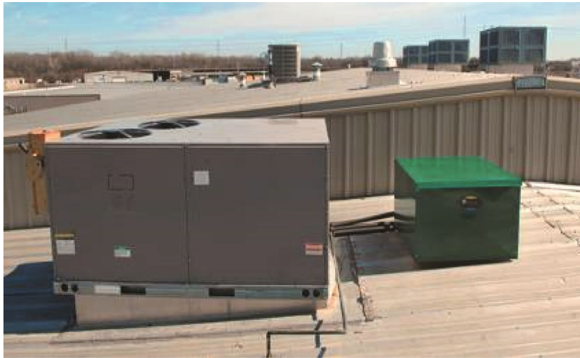
Figure 1. The equipments on the roof.
