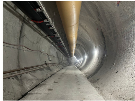
Fig. 8 Internal view of the spiral ramp with small-radius turn and steep gradient excavation (sourced from Wang et al. (2023)).
