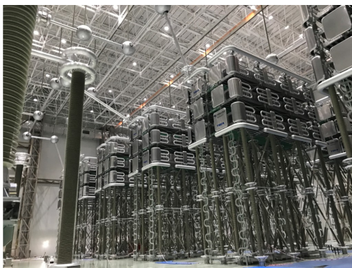
Fig. 8 The hybrid MMC valve in Kunliulong project (Liubei station).
