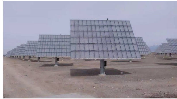
Fig. 2 Solar panel power generation unit.
