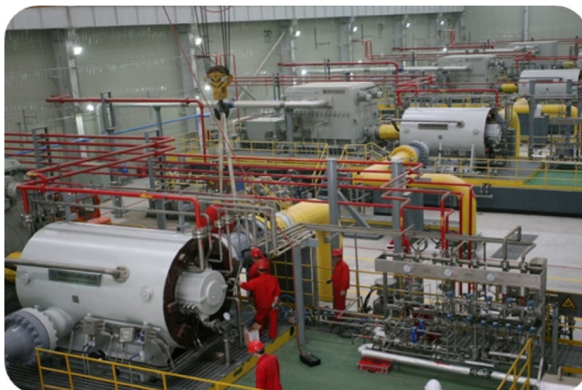
Fig. 4 20 MW electric drive compressor unit.
