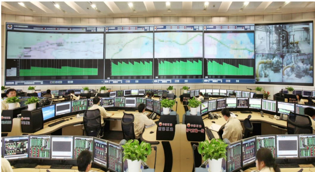
Fig. 3 PetroChina Oil and Gas Pipeline Control Center.
