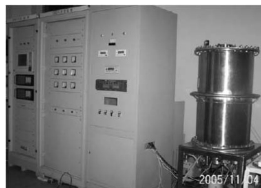
Fig. 2 Cryogenic measuring system of SMES (1. magnet, 2 & 3. radiating shield, 4. cryostat, 5 & 13. conduction strap of radiating shield, 6. magnet down conducting board, 7. flexible conducting frame, 8. cooling head conducting board, 9. cooling head of cryocooler A, 10. current lead, 11 & 15. binary current leads, 12. second stage cooling head of cryocooler B, 14. first stage cooling head of cryocooler B, 16. ice-barrel, 17. connection points, 18. digital temperature receiver, 19. computer, 20. switch, 21. digital voltage receiver, 22. digital temperature display instrument, 23. vacuum instrument)
