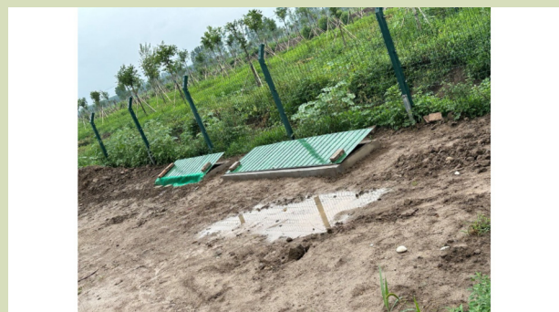
Fig. 5 Monitoring equipment after rain.
