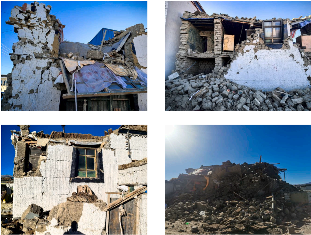
Fig. 3. Seismic damage of rural self-built houses in Changsuo Town (Intensity IX area).
