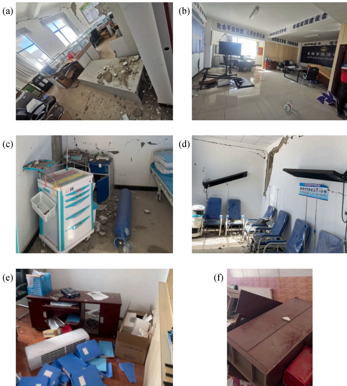
Fig. 14. Seismic damages of inside contents, (a) overturning of cabinet at town government office building in Changsuo Town, (b) overturning of projector displayer at town government office building in Changsuo Town, (c) overturning of oxygen tank and sliding of medical cart at health center outpatient building in Changsuo Town, (d) almost falling monitors at health center outpatient building in Changsuo Town, (e) falling of wall-mounted air conditioner unit and cabinet contents, and (f) overturning of cabinets at central primary school #1 teaching building of Quluo Town.
