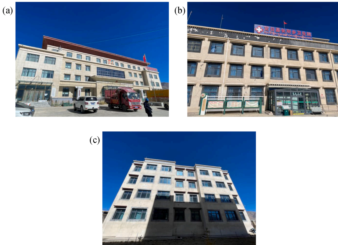
Fig. 8. Structural damages of public buildings in Changsuo Town, (a) the town government office building, (b) the health center outpatient building, and (c) the health center dormitory building.
