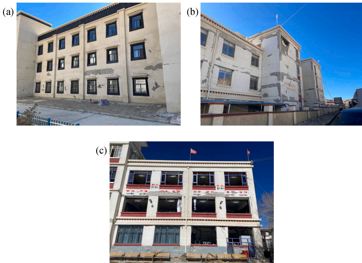
Fig. 11. Seismic damages of exterior facade walls, (a) health center outpatient building in Changsuo Town, (b) central primary school #1 teaching building of Quluo Town, and (c) central primary school #2 teaching building of Quluo Town.
