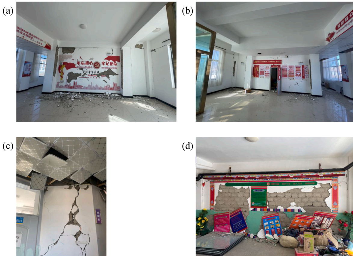
Fig. 12. Seismic damages of infilled walls, (a) spalling of plaster of infilled wall at town government office building in Changsuo Town, (b) shear cracks of infilled wall at town government office building in Changsuo Town, (c) shear cracks of infilled wall at central primary school #1 teaching building of Quluo Town, and (d) spalling of plaster at central primary school #1 teaching building of Quluo Town.
