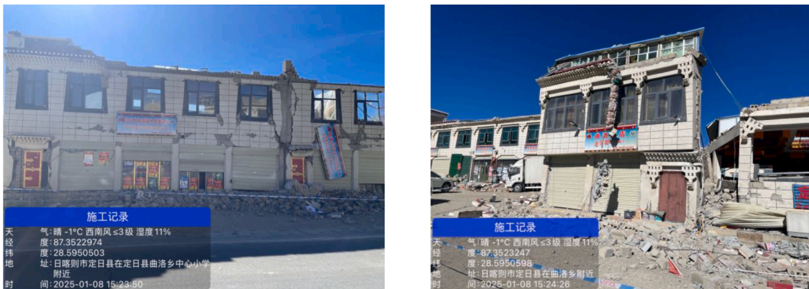
Fig. 6. Seismic damage of bottom frame structure houses.
