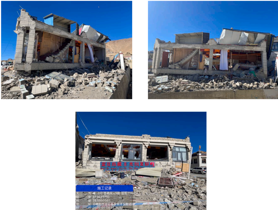
Fig. 5. Seismic damage of reinforced concrete frame houses at Quluo Town (Intensity VIII area).
