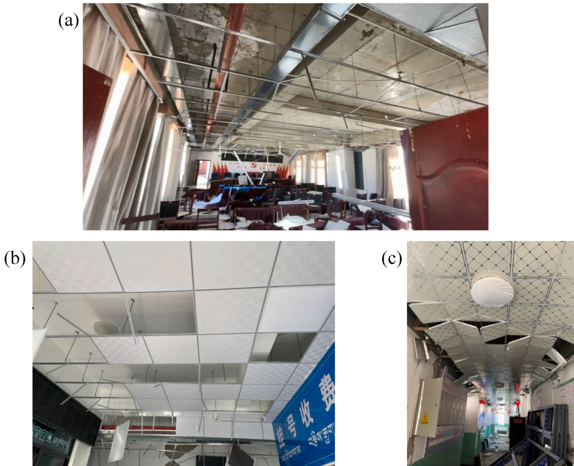
Fig. 10. Seismic damage of suspended ceiling systems, (a) government office building in Changsuo Town (Intensity IX area), (b) health clinic building in Changsuo Town (Intensity IX area), and (c) central primary school in Quluo Town (Intensity VIII area).
