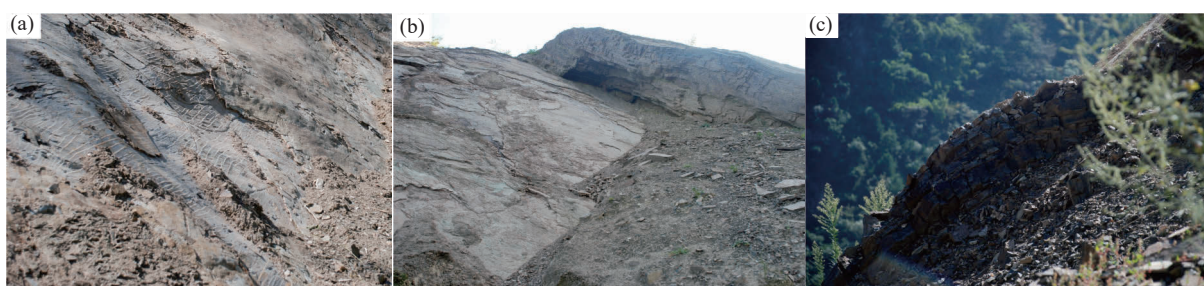
Fig. 4. Characteristics of the slip surface and shearing outlet. a–antistep in the slip surface; b–mud compounds in weak intercalation; c–bending deformation in outlet.
