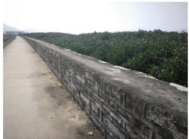
Fig. 8. The solidified seawall on the landward side of mangroves in Ningde, Fujian.
