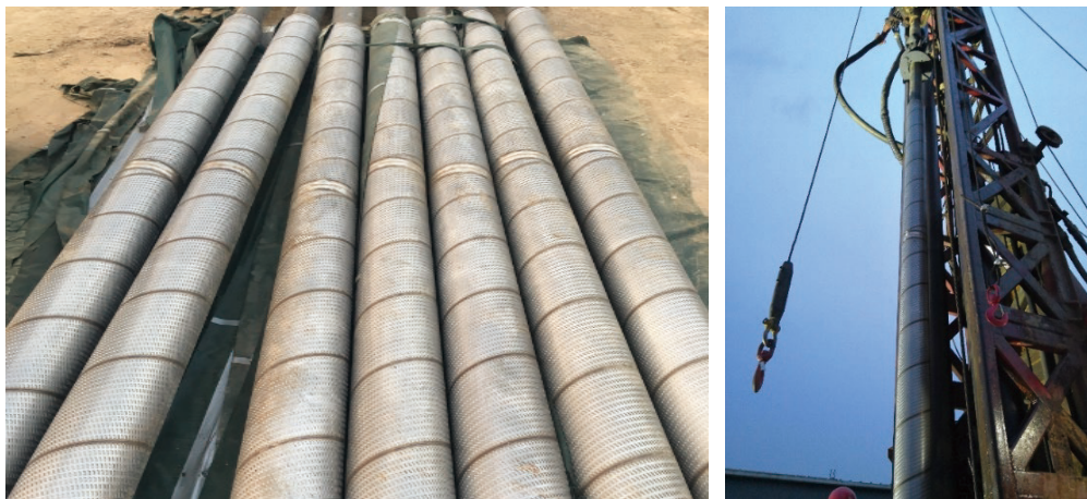
Fig. 4. Screen liner before being run into well and screen liner being run into well.
